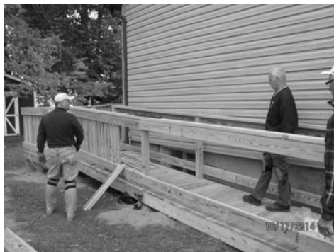
Lion's Tom, Lion Dan and Lion Bruce work to finish the ramp in late October.
